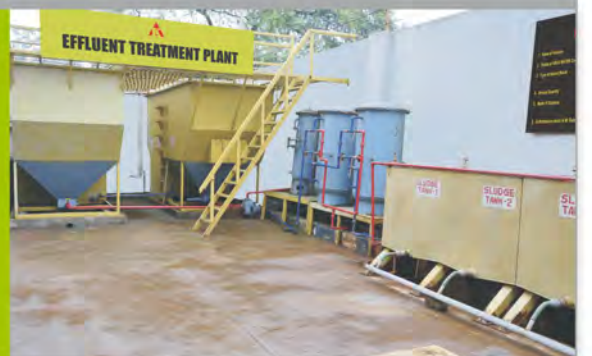
Effluent Treatment Plant
